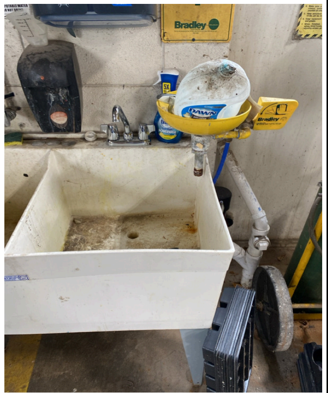
12/9/2024 - 200-34 - Malta Bend - AG Shop Double Sink - Right
