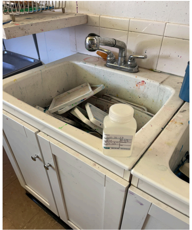
6/5/2024 - 200-30 - Malta Bend - Art Room Double Sink - Left
